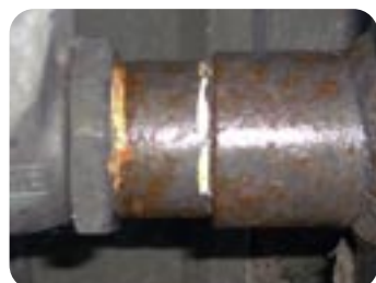
LEAKY STEEL PIPE
